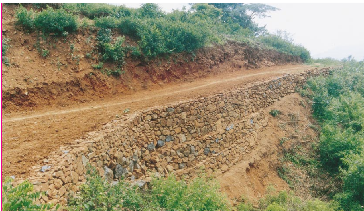
A view of the road constructed in a village of tribal area under SGRY
